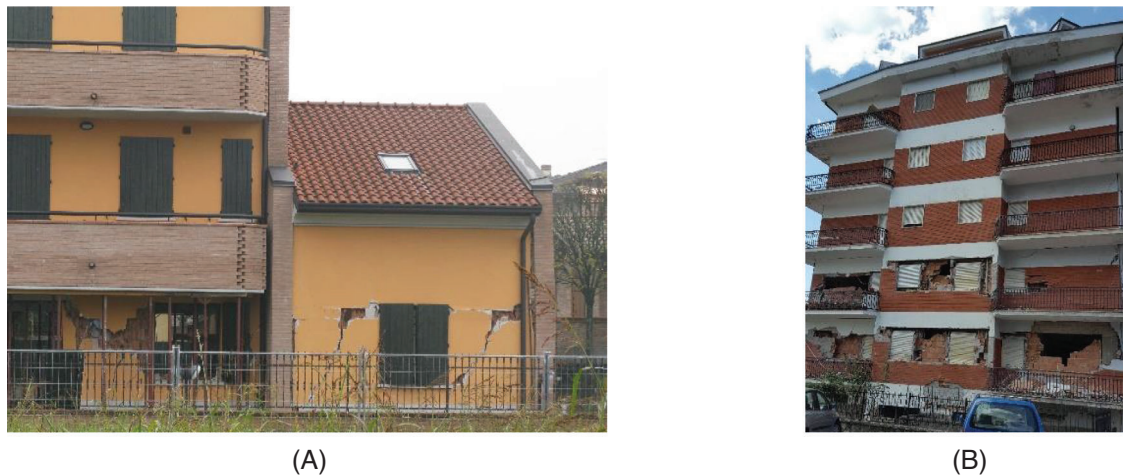
FIGURE 1 Example of earthquake damages on infills: (A) building with modern infill typology; (B) combined in-plane and out-of-plane effects
