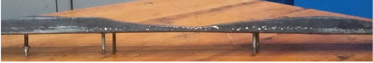
Figure 7 a) worn surface of a contact wire; b) worn thickness of a carbon contact strip.
