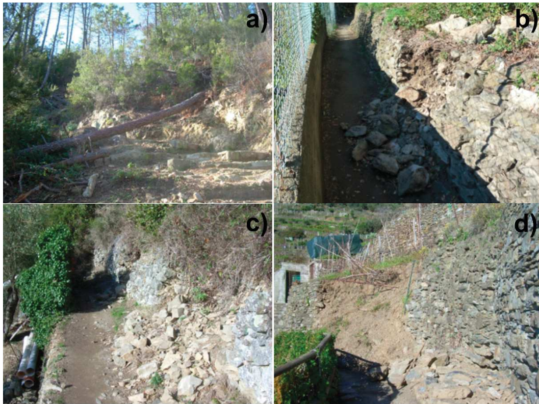
Figure 9. Examples of damage and/or rainfall-induced effects recorded using survey forms after a weather alert: (a) trees fall down; (b,c) small dry-stone wall collapses; and (d) dry-stone wall failure causing a local path interruption.
