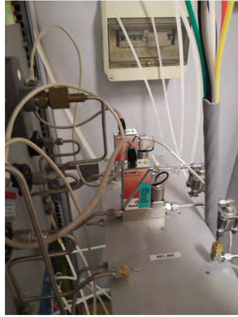
Figure 3.20: Detail of the Mass Flow Controllers used for the test.
