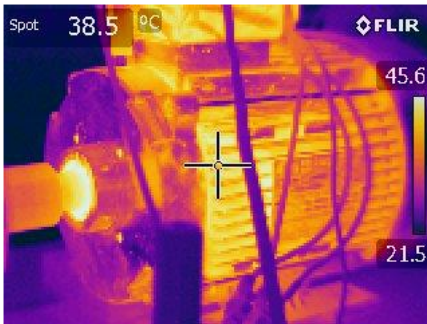
Figure 44: Thermal image of the RAEL motor with a faulty bearing in the drive-end side.
