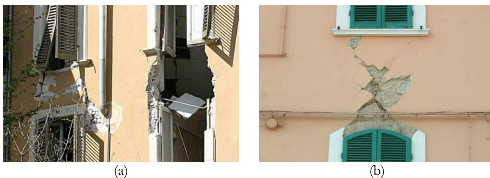
Figure 2.11: Masonry failure mechanism observation in spandrels after the 6.3 M_w 2009 L'Aquila earthquake: (a) flexural and (b) diagonal shear (Beyer and Dazio, 2012)
