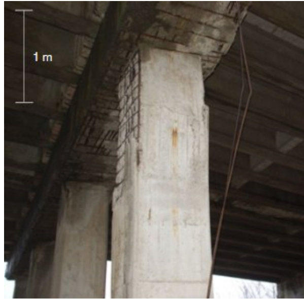
Figure 3.10. Damage on bent column with spalling of cover concrete and exposed reinforcement.
