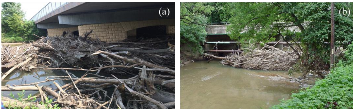
Figure 2.2 (a) A log jam spans nearly bank-to-bank in Four Mile Creek beneath Hubbell Avenue in Des Moines (Source: Timothy Meinch/The Register), (b) Peachtree Creek, Atlanta, Debris from floods cause bridge problems (Source: South Atlantic Water Science Centre).
