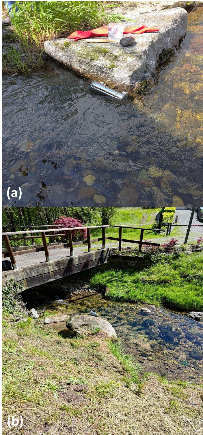
Figure 17. Installation of the HOBOT monitoring device on the Lambrone stream (a) and on the outlet stream of Lake Segrino (b).
