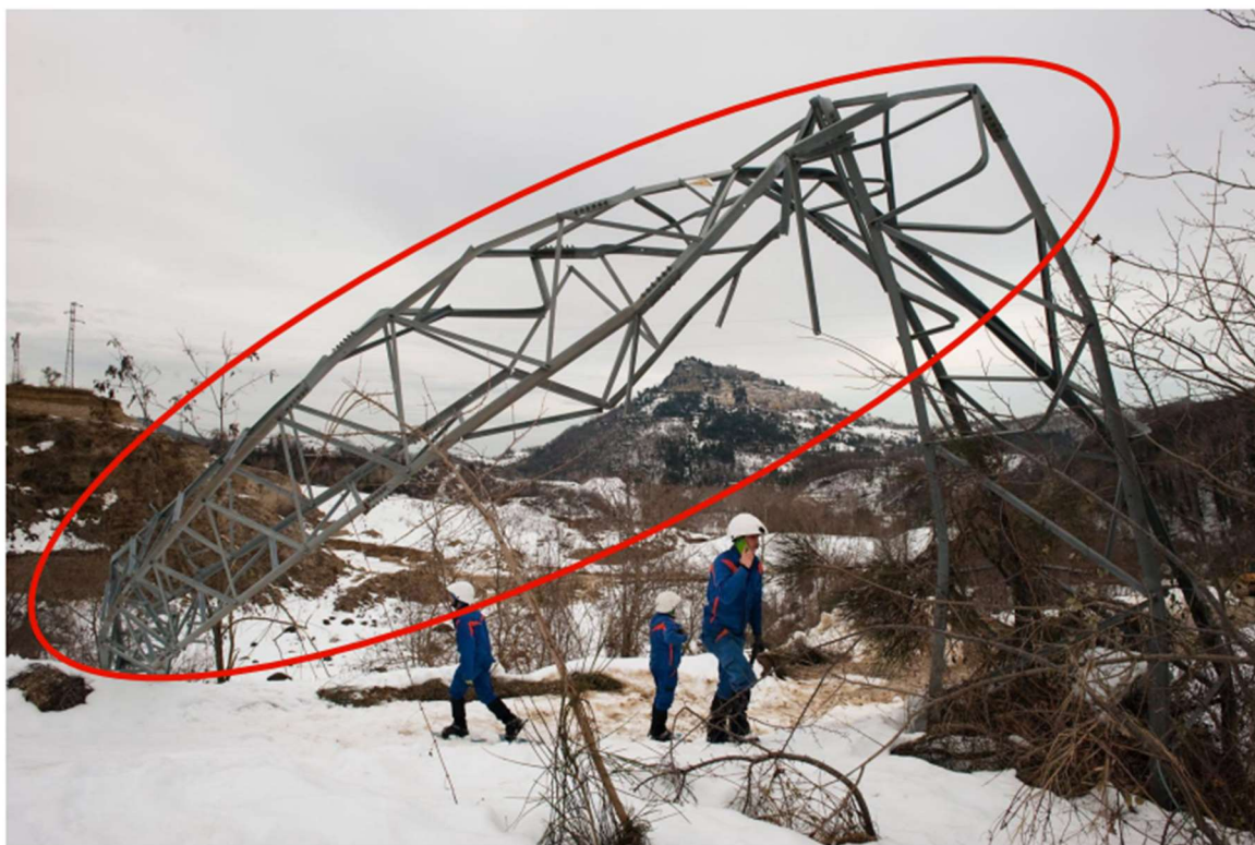
Figure 1.14 – a collapsed pole in Abruzzo, 2017
