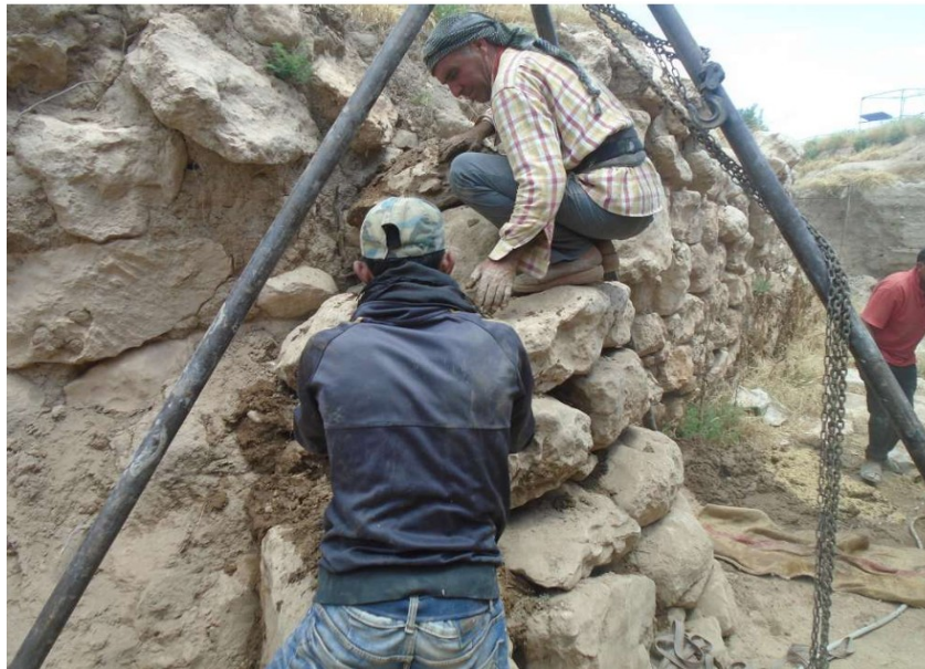
Figure 55: The construction process of the retaining wall in Area J5 of the temple. Personal photograph by the author, 2019.
