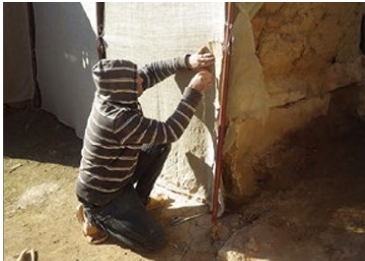
Figure 59: The routine maintenance work on the burlap covering in the palace area. Source: Buccellati. 2019, 194.
