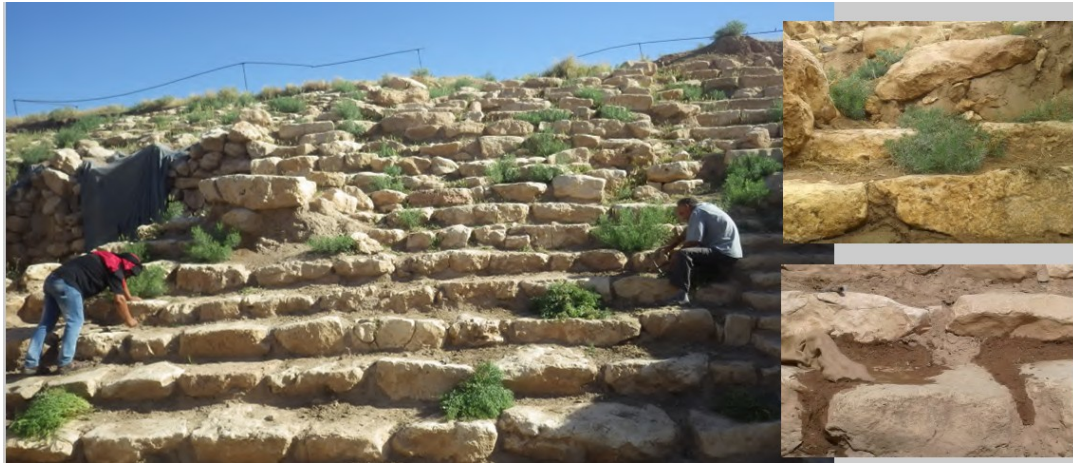
Figure 52: The application of clay mortar between the stones after removing weeds, with the newly applied mortar covered by a piece of fabric placed over the old mortar on the staircase of the temple. Source: Buccellati et al. 2019, 3.
