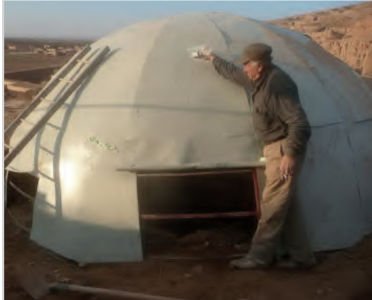
Figure 50: The new dome completed, with openings at the base. Source: Buccellati et al. 2018, 36.
