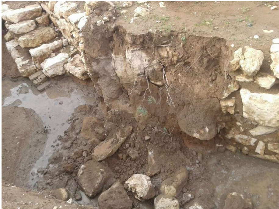
Figure 53: The collapsed retaining wall in Area J5 of the temple. Personal photograph by the author, 2019.
