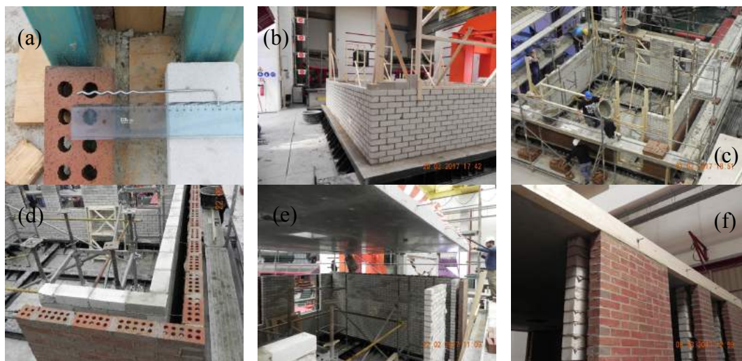
Figure 3.3 Construction details of the specimen: (a) geometry and positioning of cavity steel tie; (b) building phase of inner CS leaf; (c) construction of the ground floor; (d) inner and outer leaves before the laying of the RC slab; (e) laying of the first-floor slab; (f) connection of slab to longitudinal walls and timber plate.
