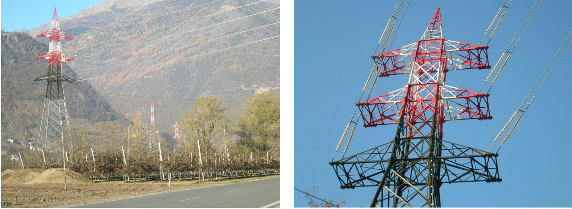
Figure 3.4.2: A 380 kV voltage power transmission line under construction in Valtellina, Alps, Northern Italy [Credits: Gianmario Rinaldi].
