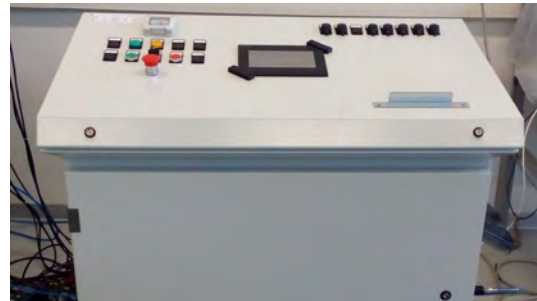
(b) electrical cabinet
